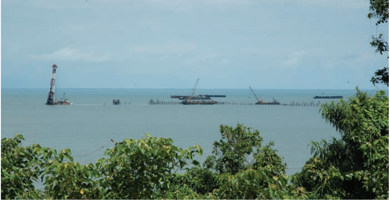
PLATE 1 | Offshore construction phase activities of the BP Tangguh LNG Project (Papua, Indonesia). A construction phase exclusion zone excluded both fishing activities within the area and passage of fishermen through the area, thereby restricting their access to other fishing grounds. Ships involved in supply of goods and services laid anchor outside the exclusion zone representing additional hazard and disruption to fishing activities and transit through the area. A larger exclusion zone came into force during the operations-phase of the project. Credit: Robert Gerrits
